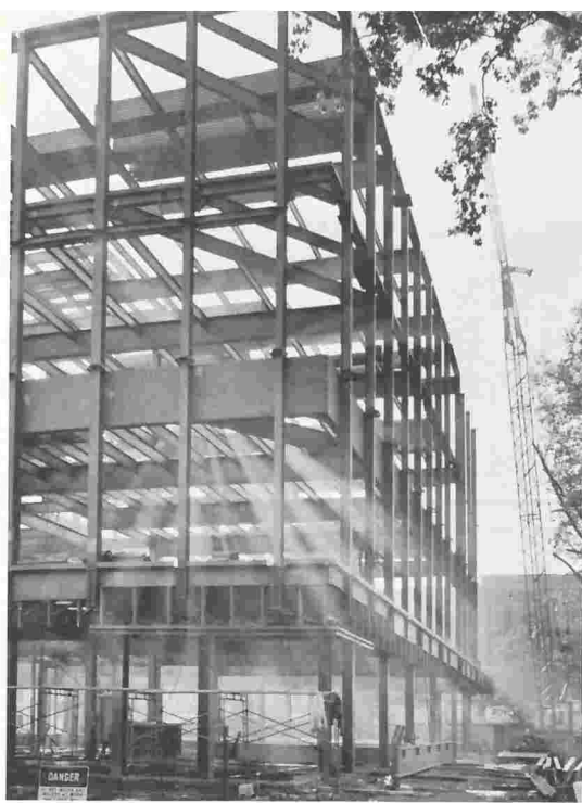
The steel skeleton for the new building took shape in October 1969. In winter it was shrouded with heavy plastic and . . .
